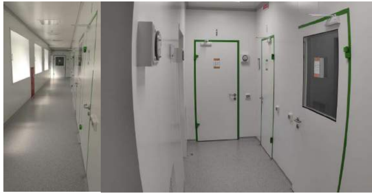
Technological corridor of clean rooms (class C, D)
